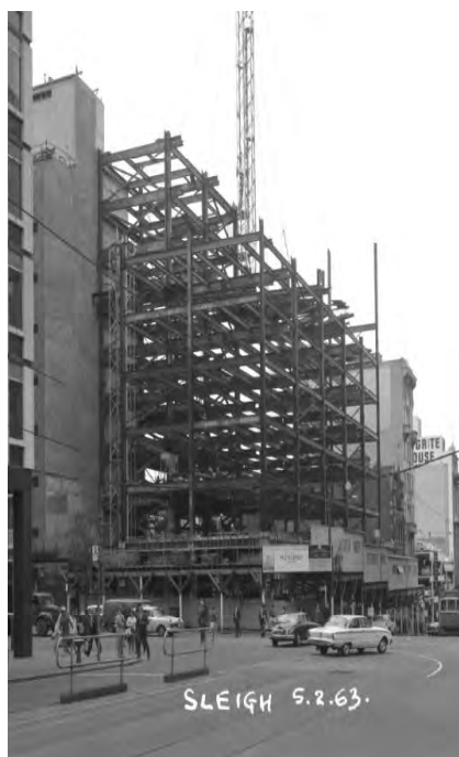
Figure 3. The subject building during construction. The sign on the scaffolding is advertising the site as the new headquarters for H C Sleigh. (Source: Sievers 1963, NLA)
