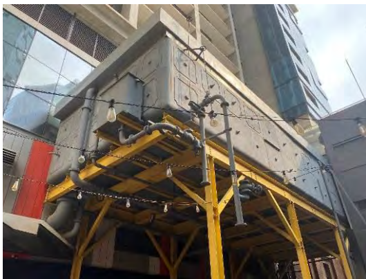
Figure 14. The Overhead Water Tank, built 1888 and relocated to this site in c1927. (Source: Context, February 2020)
