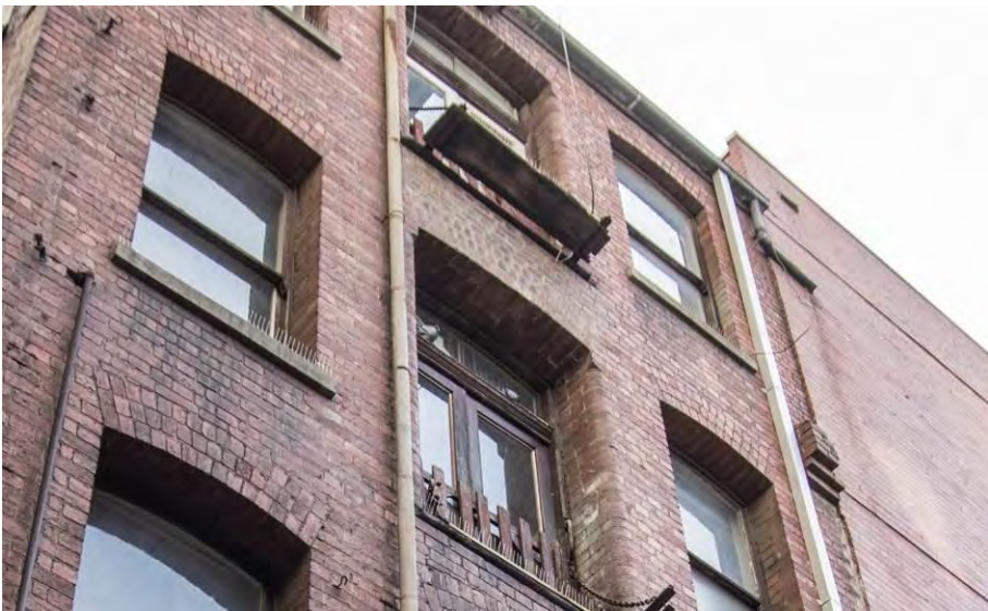
Figure 22. Note the remnant corbelled bracket on the northern (RHS) edge of the second floor of 3 Kirks Lane. (source: Context, January 2019)
