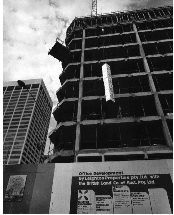
Figure 5. The building under construction in 1974. The site board states that the office development was by Leighton Properties Pty Ltd with The British Land Co. of Aust. Pty Ltd, and that construction started in April 1973 (SLV, Wolfgang Sievers, photographer, Image H99.50/384).
