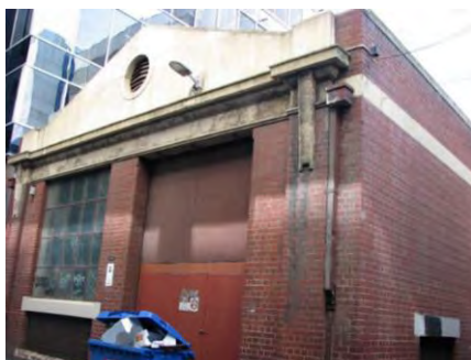
Figure 8. Substation, 10-14 Park Street constructed 1928. (Source: Context 2017)
