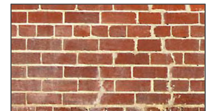
HT4- ORIGINAL EXPOSED BRICK (IF DEEMED POSSIBLE) WITH FEATURE ELEMENTS IN LIGHT RENDER
