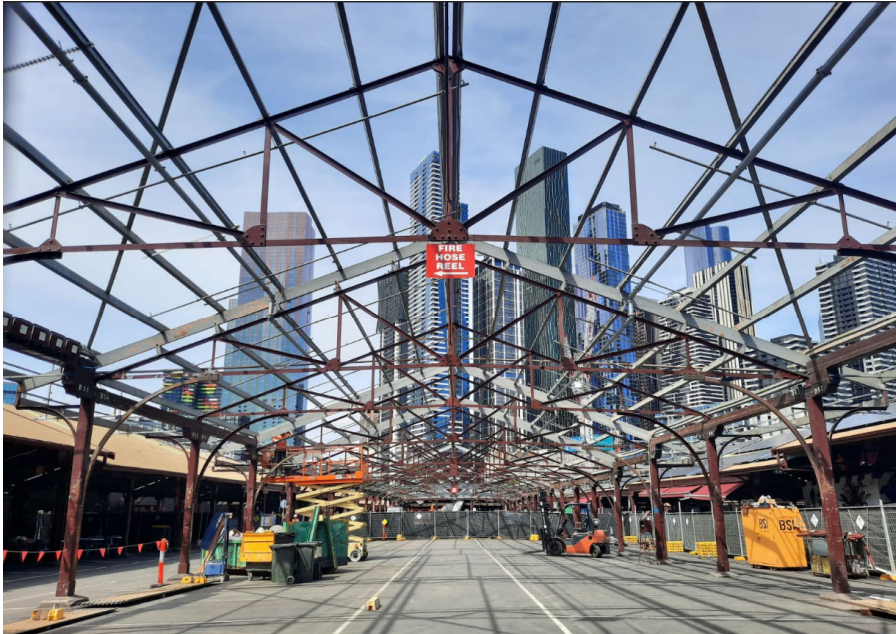
Figure 1 – Shed D, looking towards Queen Street from Peel Street end with the site prepared for the installation of new thermal roofing.
