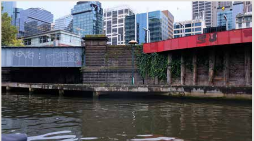
↑ ... poorly maintained assets in need of renewal ...
