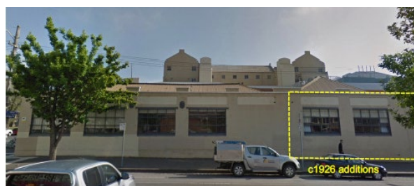
Recent photograph of the Pelham Street elevation. The dashed line marks the 1926 extension
