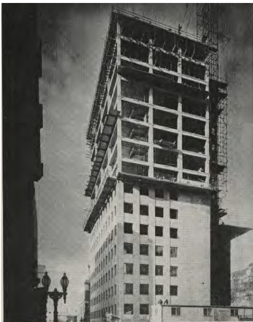
Figure 4. Image of the building under construction, published in the August 1965 edition of Cross-Section as part of an
