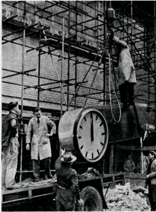
Figure 4. Extract from photograph showing the 6cw (approximately 300kg) timepiece being installed at Russell Street Exchange building in 1954. (Source: Age 23 July 1954:8)
