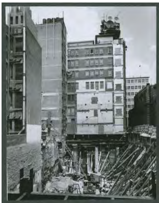
Figure 5. Excavation for the Lonsdale Telephone Exchange showing the back wall of the 1937 City West Telephone Exchange building. (Source: NAA 1966: series B6295, item: 1609B )
