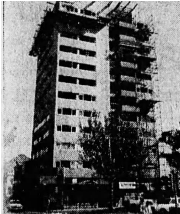
Figure 4. Image of the building under construction, published in May 1970 in a sales advertisement for the units ( Age , 2 May 1970:39).
