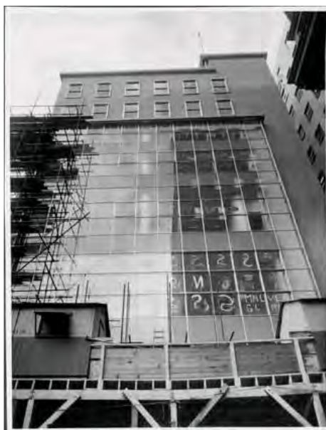
Figure 2. The subject building at completion c1957. (Source: NAA 1957-1984, Series: B6295, Item no: 9723653)
