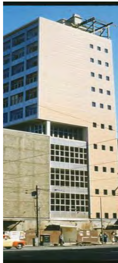
Figure 7. The construction phase. Photo probably dates to 1955-56 (SLV, Peter Wille, photographer, Image H91.244/3970).
