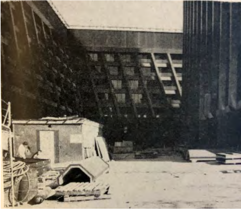
Figure 6. The buildings under construction, image published in the May/June 1969 edition of Architect .
