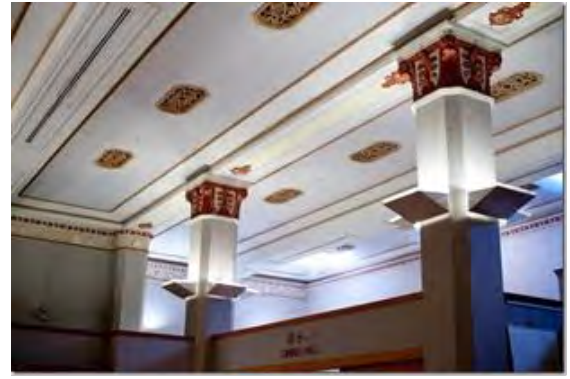
Figure 10. Ground level chamber ceiling and column detail ceiling. (Source: Melbourne Heritage Action)
