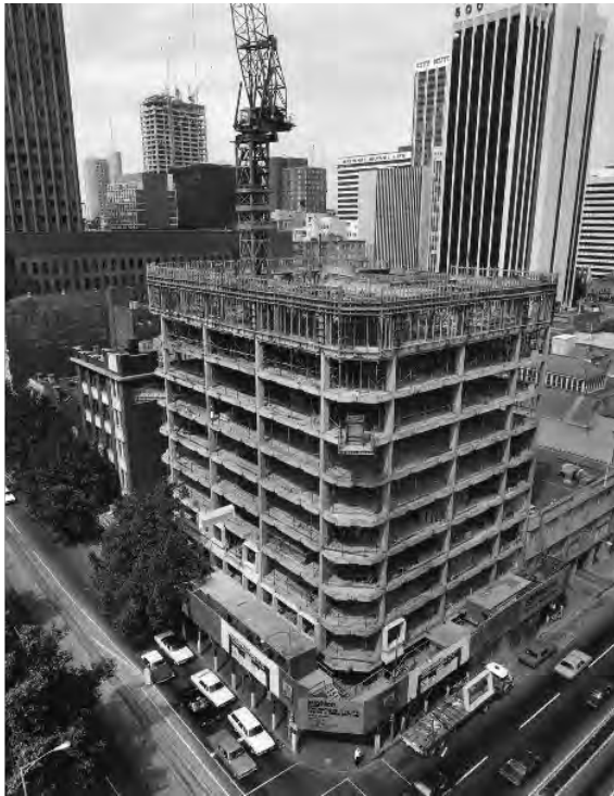
Figure 4. The corner building under construction in 1974 (SLV, Wolfgang Sievers, photographer, Image H99.50/383).
