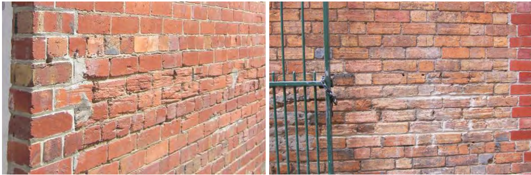
Figure 6. Vehicle marks on 27-29 Little Lonsdale (left) and a neighbouring building at 23-25 Little Lonsdale Street. (Source: Context 2018)
