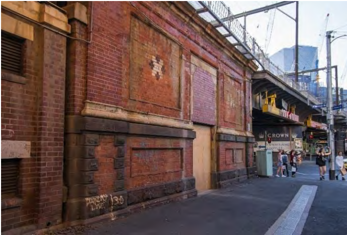
Figure 18. Close up of the undercroft (perhaps part of the 1890s construction). (Source: Context 2019)
