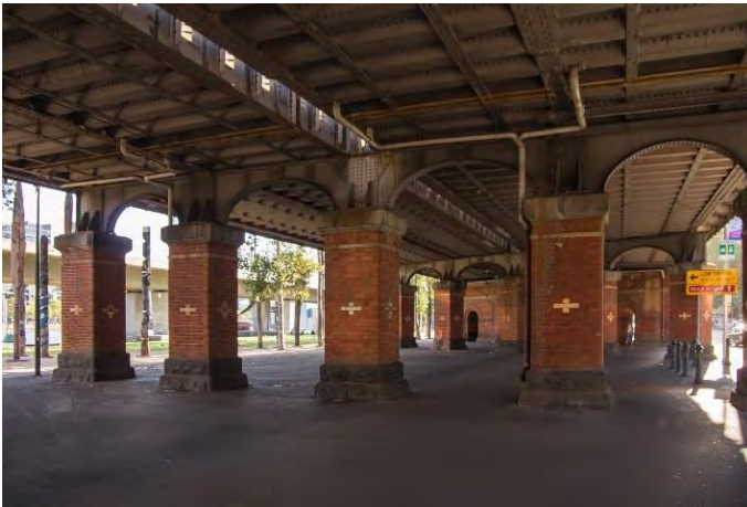
Figure 13. View towards west, near intersection of William and Flinders streets. Three piers on the left-hand side are from 1891 and one on the right-hand side is from 1917. (Source: Context 2019)
