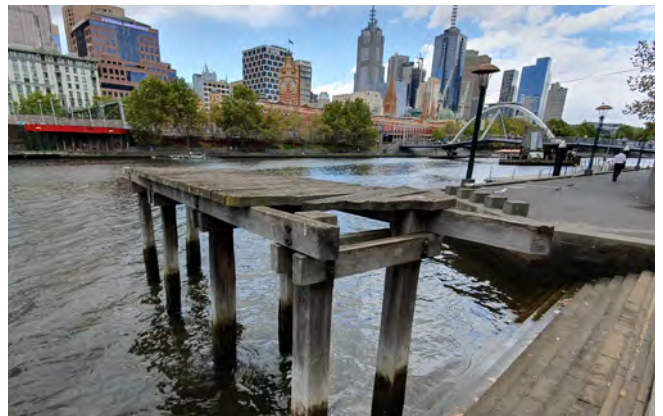
Image 44. Broken Pier, Southbank Spillway
