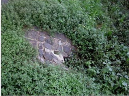
Outfall drain and stone apron at north end of Moonee Ponds Creek section, may contain early stone work
