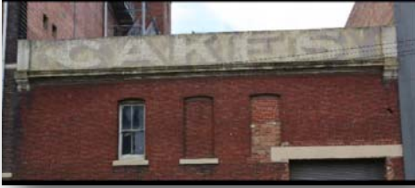
Figure 24 parapet sign Building 10 -Part TB Guest complex, Laurens
