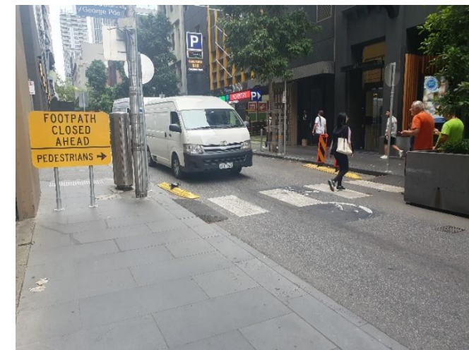
Example of a temporary zebra crossing installed for construction (Flinders Lane, Russell to Exhibition)
