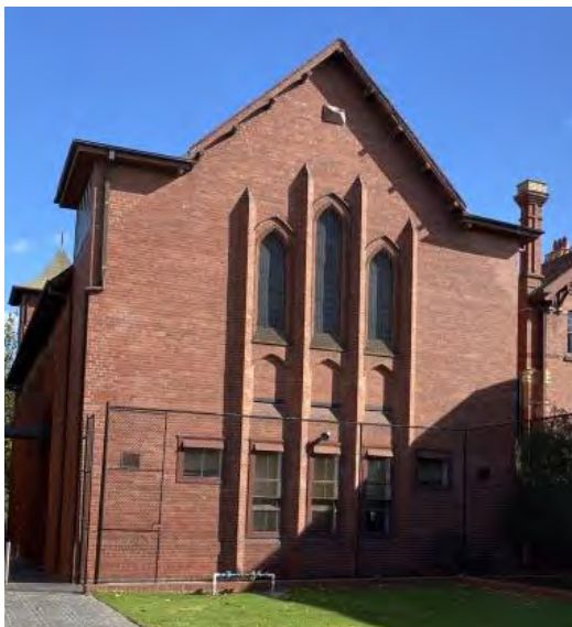
Figure 13. Rear façade of the chapel, facing east. The addition of dormer windows has changed the profile of this roofline, evident in the two horizontal projecting rooflines shown in this picture. (Source: GML Heritage 2021)
