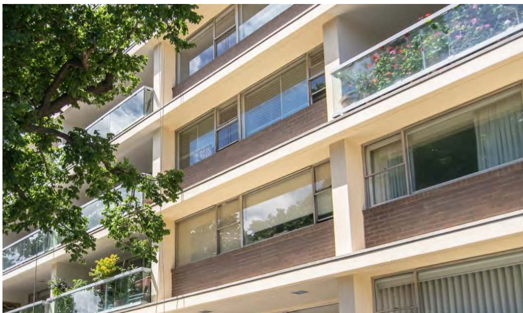
Figure 2. Section of the primary elevation in 2020, showing the intact original detailing. (Source: GML Heritage 2021)
