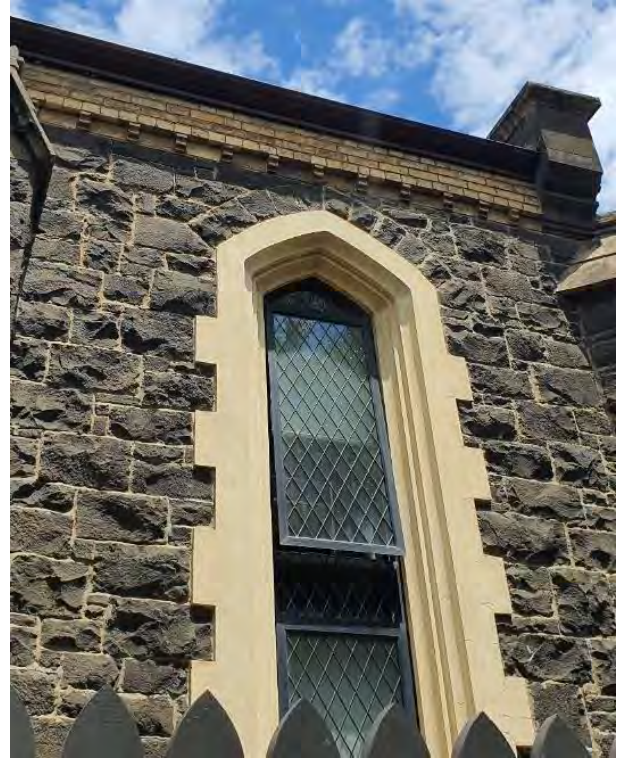
Figure 7. An opening on the north elevation, with cement rendered edges and replacement diamond pattern window. (Source: GML Heritage 2021)
