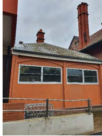
Figure 18. Image showing the slate clad roof and chimney and the enclosed verandah. (Source: GML Heritage 2021)
