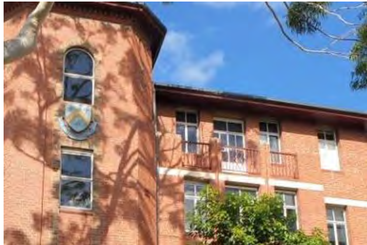
Figure 16. Detail showing dark brown brick detailing and mild steel balcony balustrade. (Source: GML Heritage 2021)
