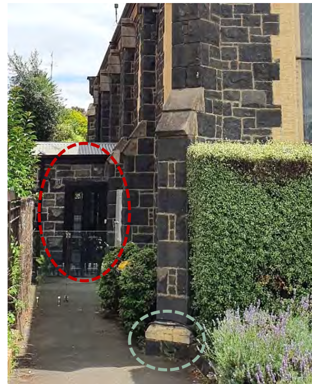
Figure 9. View of the south elevation, showing the bluestone addition that most likely dates from c1994 (outlined red) and the burnt white clay water table (outlined yellow). (Source: GML Heritage 2021)
