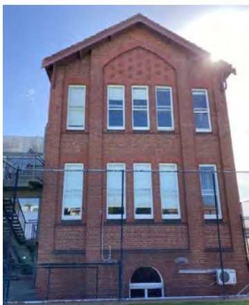
Figure 9. Photograph showing part of the southern façade of the rear extension. The terracotta tile detailing on the gable end is visible. (Source: GML Heritage 2021)
