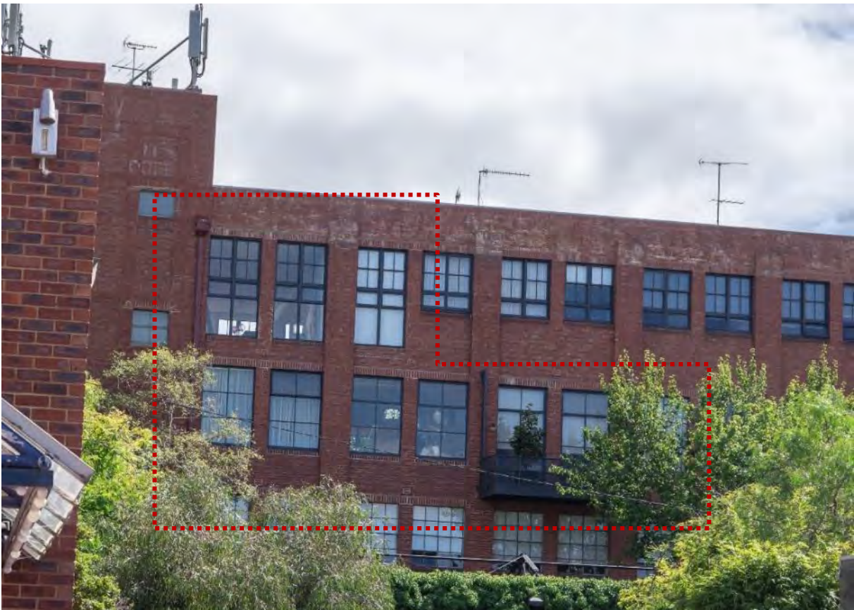
Figure 14. South elevation of the 1922 former storage building, showing the altered window openings on the second and third floors (in dashed lines). The first-floor level window openings and frames appear original. (Source: GML Heritage 2021)
