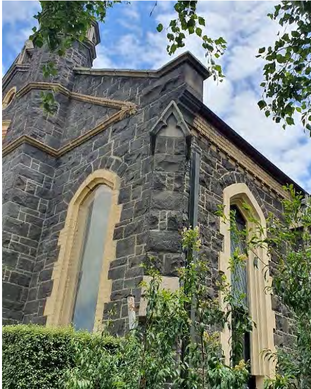
Figure 6. Close-up view of detailing, including the cement dressing on the buttress, moulded cream brick stringcourse and quoining (left), cement rendered quoining (right). (Source: GML Heritage 2021)
