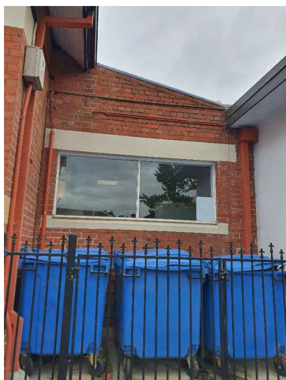
Figure 14. Skillion roofed hat and cloakroom 1923–24 extension with aluminium-framed windows. (Source: GML Heritage 2021)
