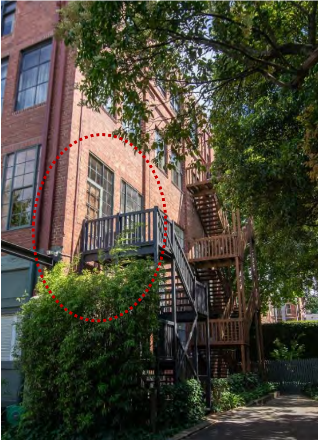
Figure 17. On the east elevation of the 1922 former storage building, some windows are extended with new window frames. Altered window openings are shown in dashed lines. Timber stairs on the east elevation are later additions that are sympathetic to the former industrial character. (Source: GML Heritage 2021)
