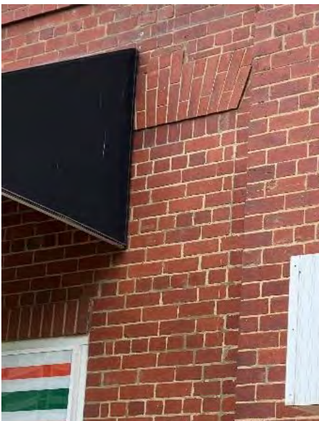
Figure 11. Evidence of original window openings on the ground floor. (Source: GML Heritage 2021)
