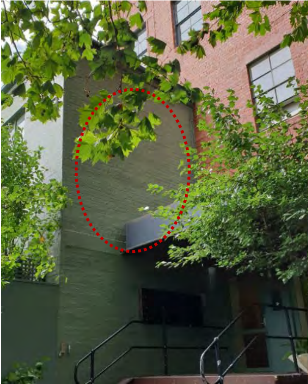
Figure 13. Face brick (now overpainted) former grain store building, built c1889, adjoining the main building. The original openings on the south elevation shown here are now bricked in (outlined in red). The entrance and the steps are additions from 1978 (Source: GML Heritage 2021)
