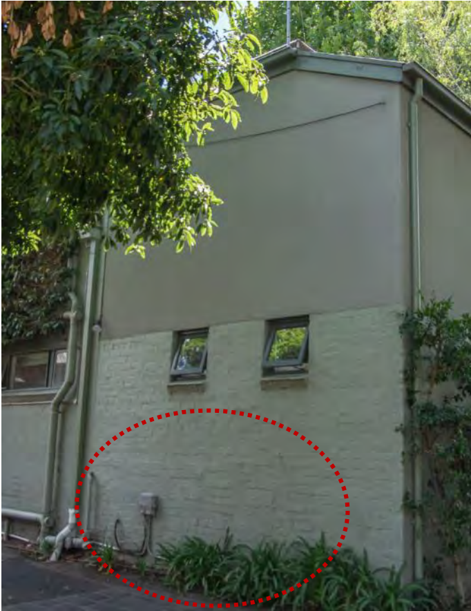
Figure 19. The face brick (now overpainted) lower section of the former toilet block likely dates to c1889. The original segmental arched openings on the south elevation are bricked in (outlined in red). The new windows above are not original. (Source: GML Heritage 2021)
