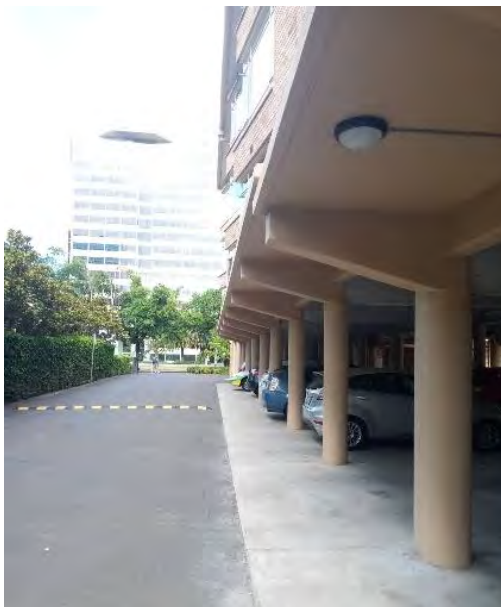
Figure 11. Cantilever from pillar to first floor base on the southern side. (Source: GML Heritage 2021)
