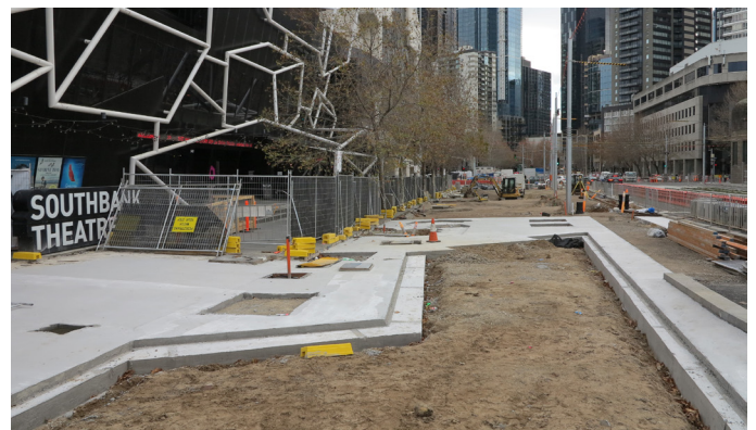
Concreting works in the landscape space to the front of the Melbourne Recital Centre are now close to complete.
