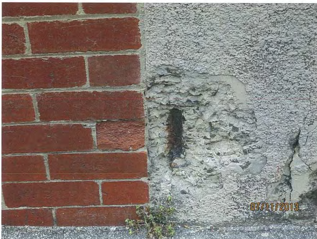
Expansive brickwork spalling. Spalling concrete due to steel corrosion.
