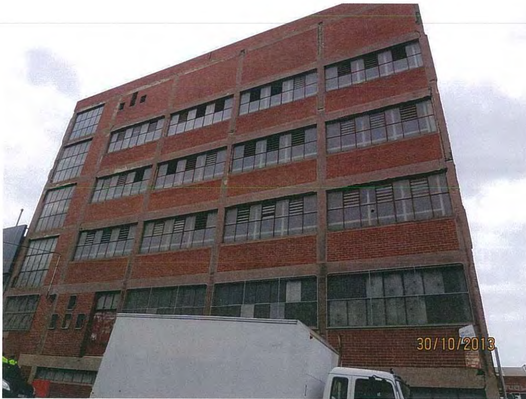
Northern elevation spalled concrete from columns and beams. Hoarding or gantry required.
