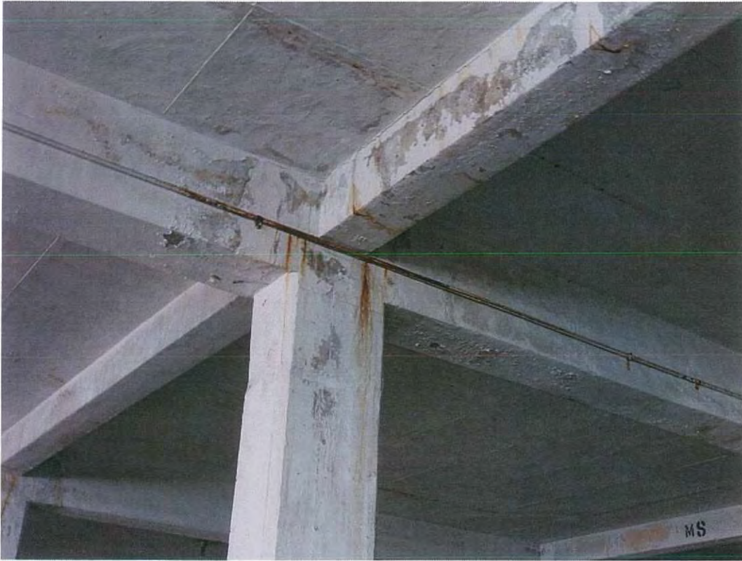
Internal concrete framework showing corrosion of reinforcement due to low strength concrete and moisture ingress into building
