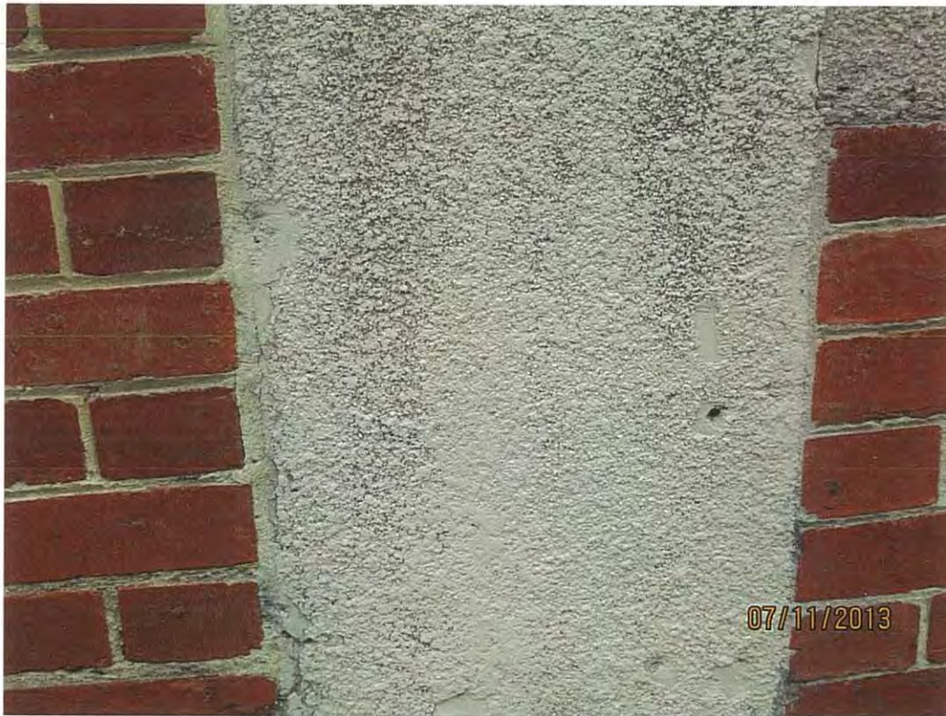
Solid mortar joints – no allowance for expansion
