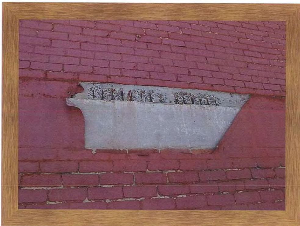
Spalling of Southern façade
