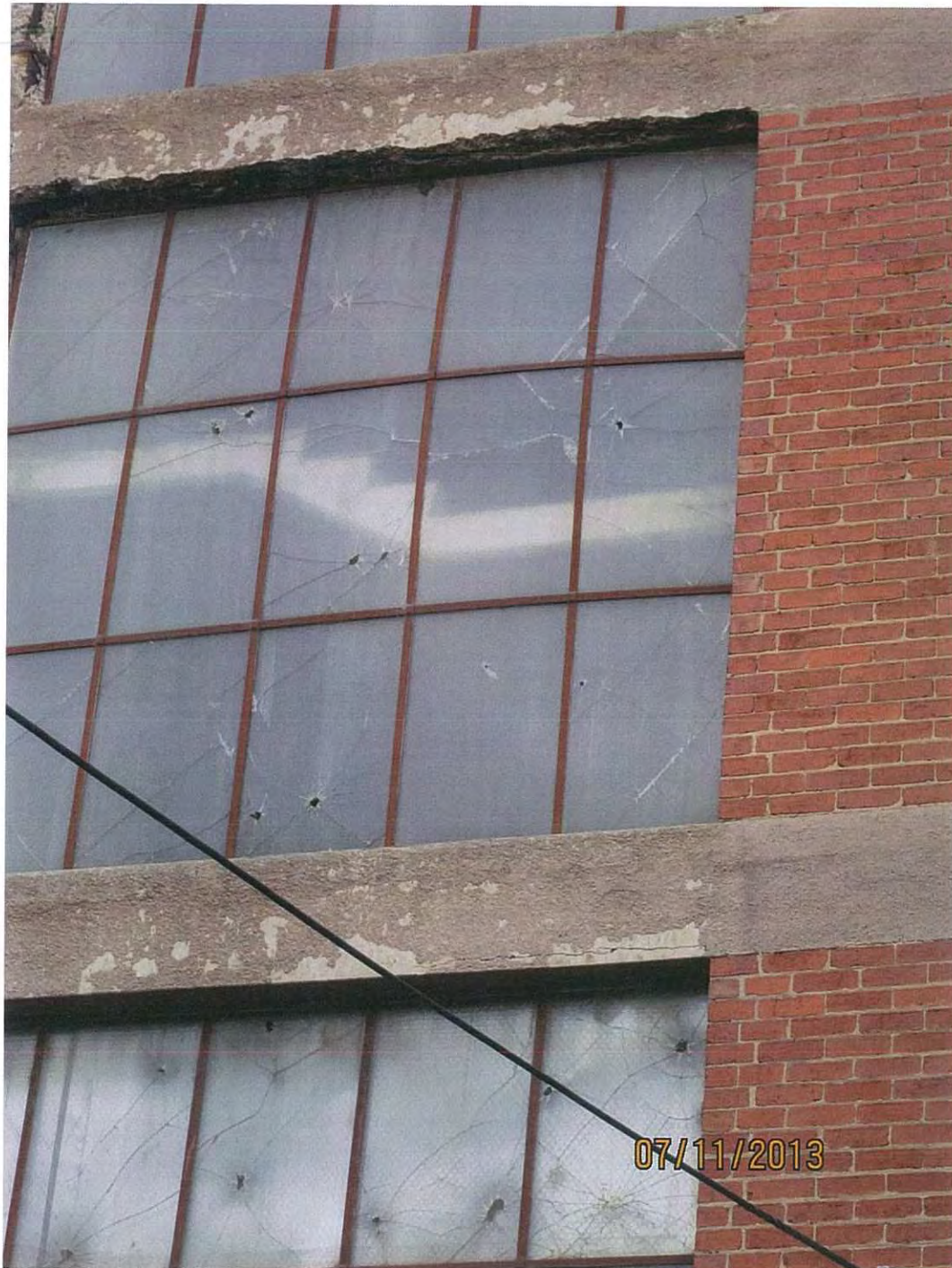
Steel window framing bowed. Glazing breaking into shards. Will fall on footpath.
