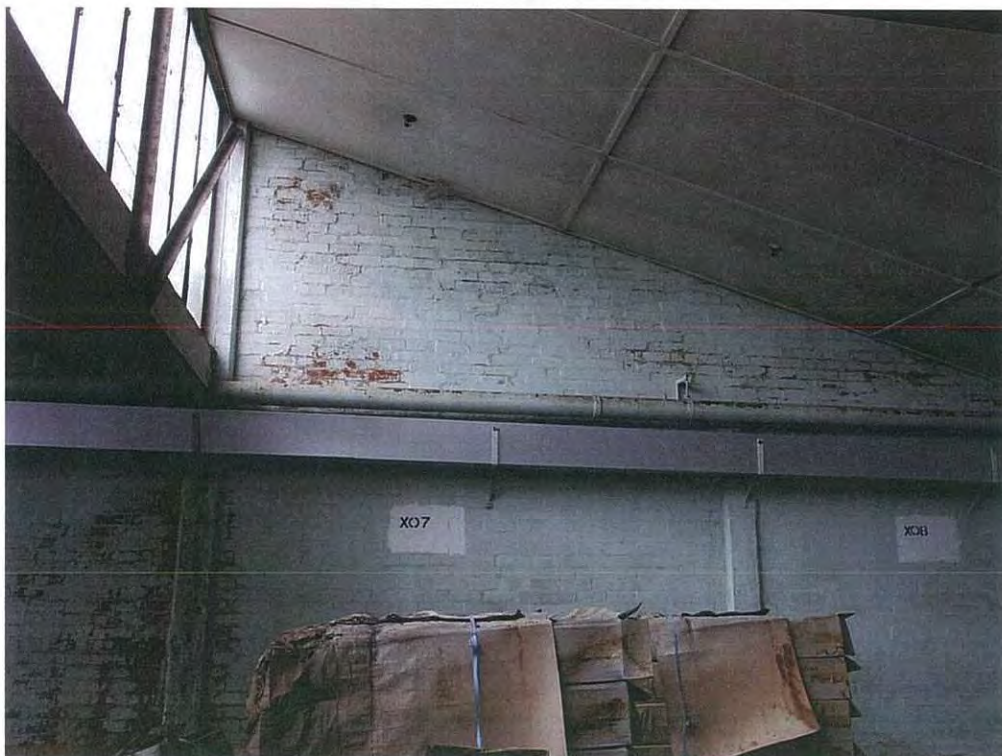
Expansive bricks in sawtooth brickwork require complete replacement
