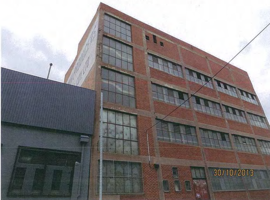
Northern elevation spalled concrete from column. Hoarding or gantry required.
