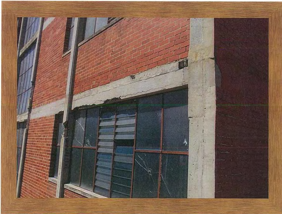
Western façade – corrosion of steel window frame and cracked window panes. Spalling concrete lintel
