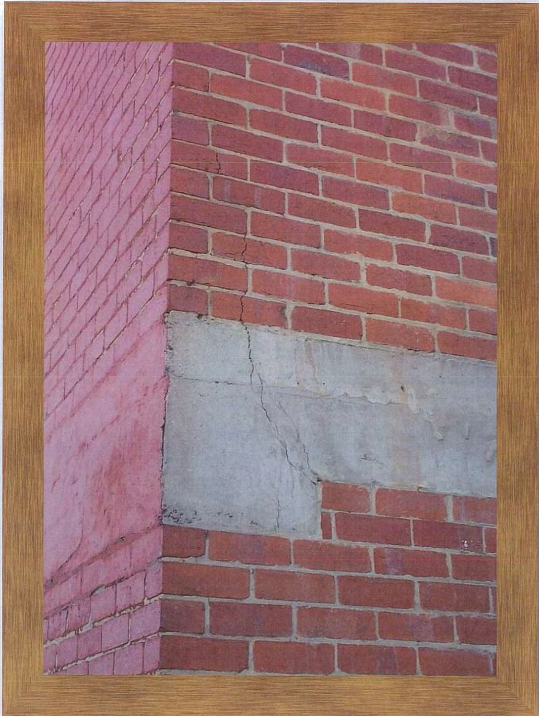
Eastern elevation – no expansion joints – brick expansion causing cracking of brickwork and perimeter beam
