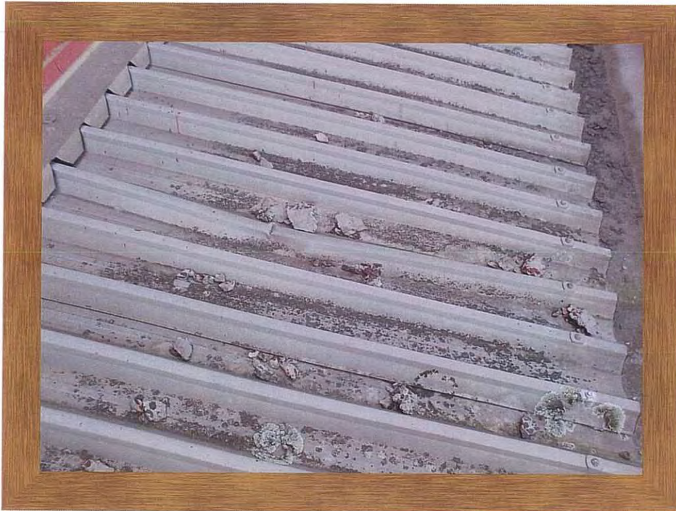
Spalls from Southern façade onto adjacent building
