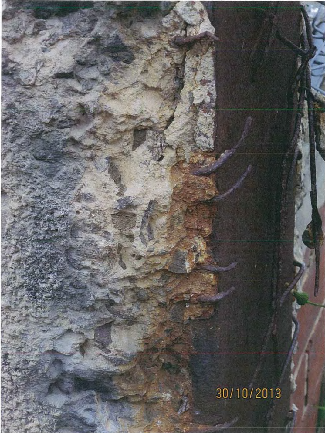
Severely corroded steel column. Failed reinforcement and spalled concrete. Inadequate cover.
