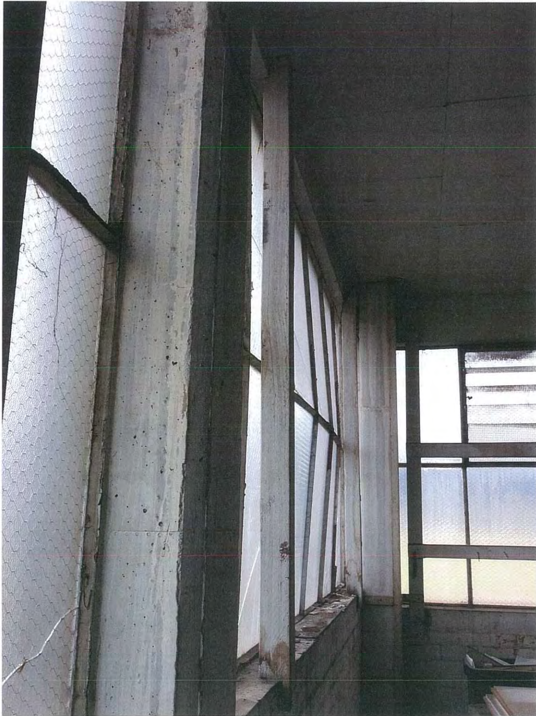
Bowing window frame causing glazing to break into shards
