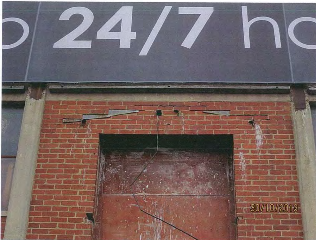
Spalling of concrete on steel columns and failed brickwork.
