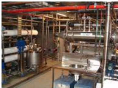
Figure 3: CH 2 sewer mining plant
