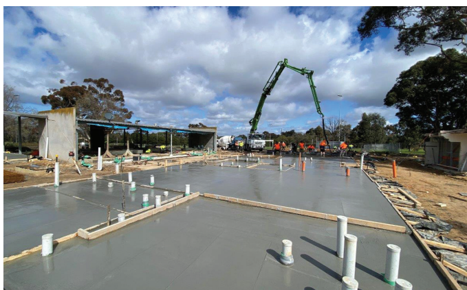
Concrete slab and pipe works in the middle section of the pavilion
