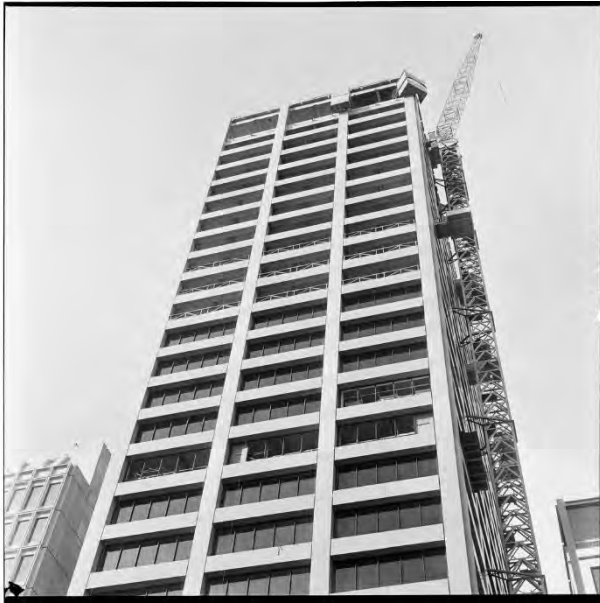
Figure 6. The tower under construction; photo dated c1975 (SLV, Hans Bonney, photographer, Image H2009.50/262).
