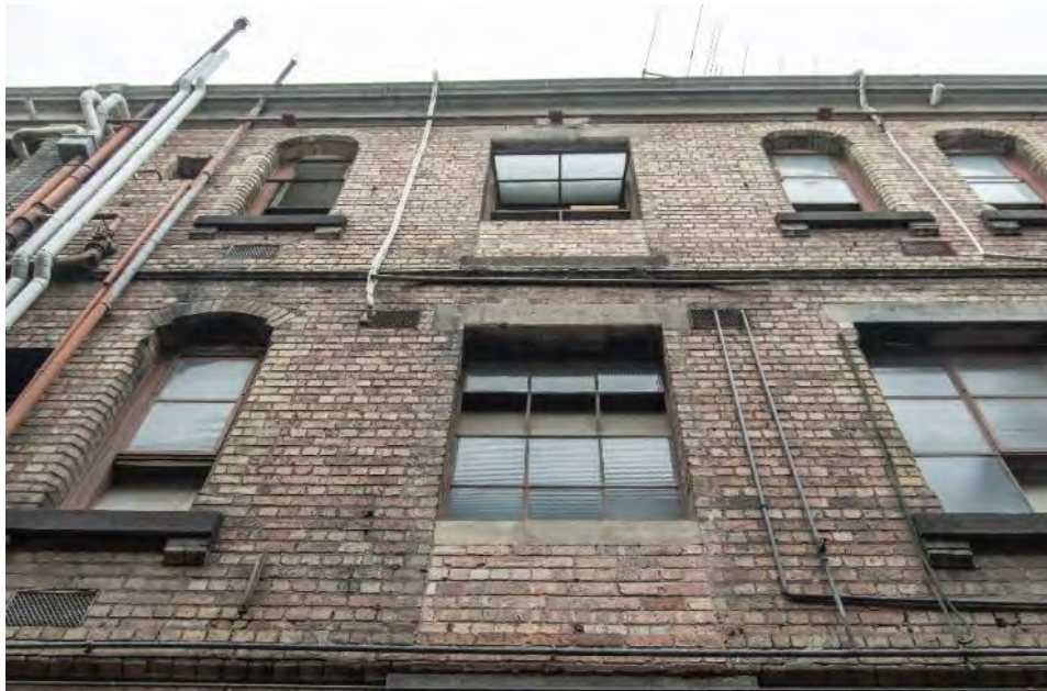
Figure 8. Side elevation of 365-367 Little Bourke Street fronting Warburton Lane. Later rectangular openings with concrete lintels and sills, and the original window openings with cement sills with brackets and splayed edges on the either side of the later openings. (Source: Context, January 2020)
