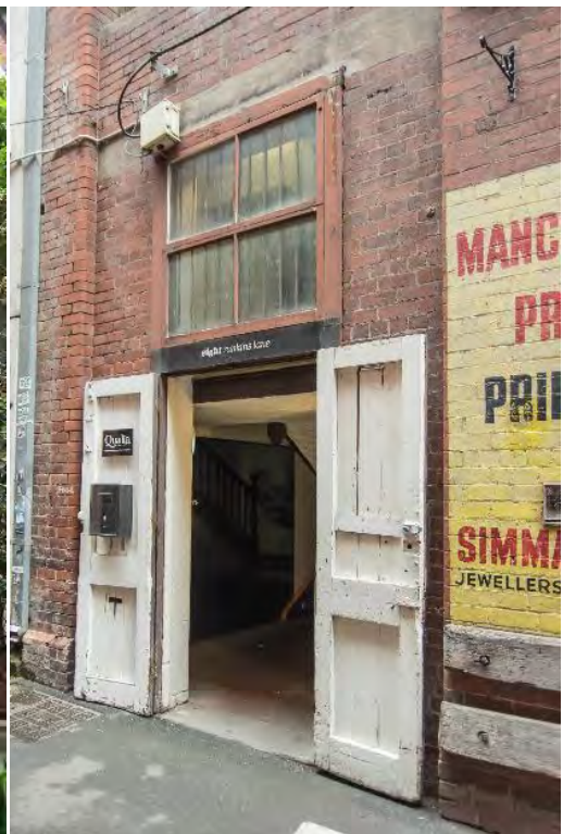
Figure 12. Example of intact openings and timber doors and windows at 8-14 Rankins Lane. (Source: Context, January 2020)
