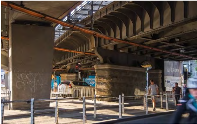
Figure 19. Spencer Street tram stop. Concrete piers dating from the 1970s, and the bluestone pier from 1917. (Source: Context 2019)
