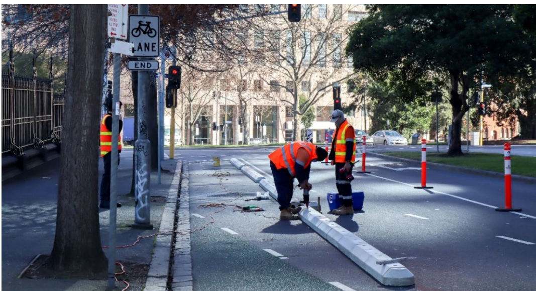
Figure 3: Workers install Orca protective kerbing to improve the quality and connectivity of the bicycle network in Albert St East Melbourne Source: City of Melbourne
