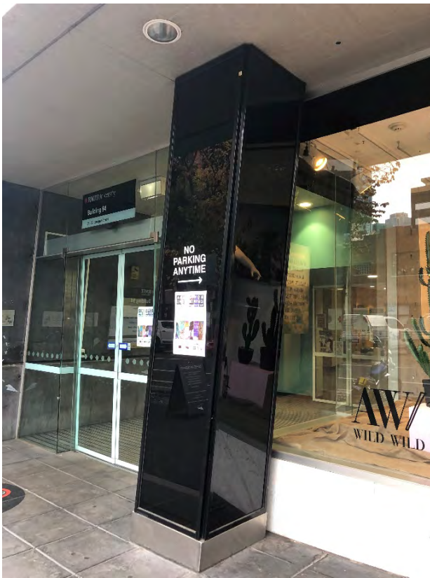
Figure 13 Detail of tilted column, recessed ground floor to northern bay Source: Lovell Chen
