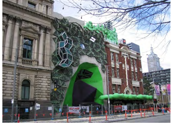
Figure 15 Storey Hall, 336–348 Swanston Street, Melbourne, H1498 and HO482 Source: The Red and Black Architect
