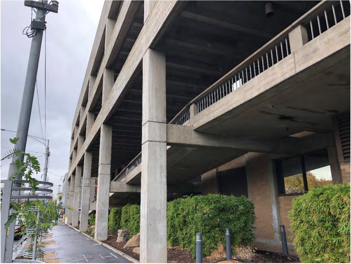
Figure 10 Detail of the concrete ramp, and its underside, which comes up from the east end of the building (in the distance) within the double-height colonnaded loggia Source: Lovell Chen
