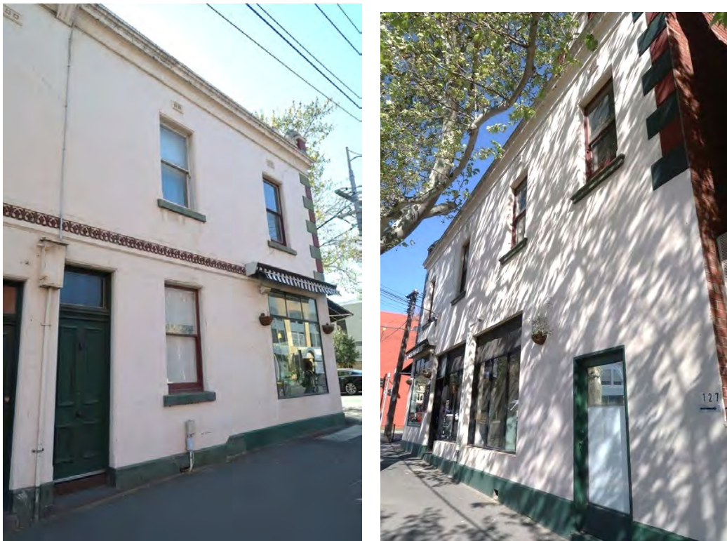
Figure 8 Nos 83-87 Cardigan Street; Cardigan Street façade (at left); Queensberry Street facade (at right) Source: Lovell Chen
