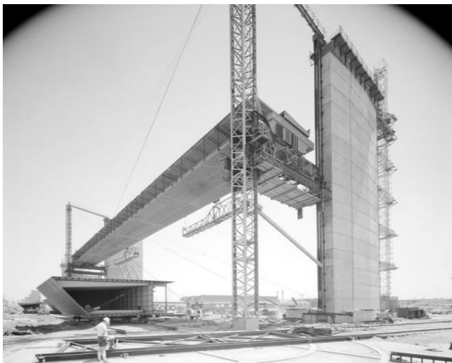
Figure 8: Lifting of a box girder during construction (Laurie Richards Studios, 1969, MOV Item MM 55221)
