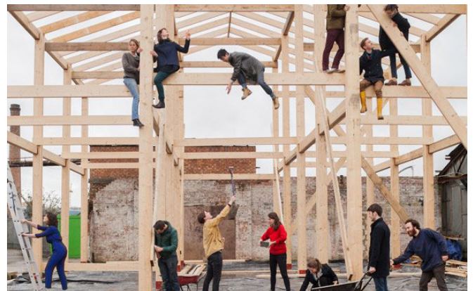
Image of Assemble building the Yardhouse in London courtesy and copyright of Assemble
