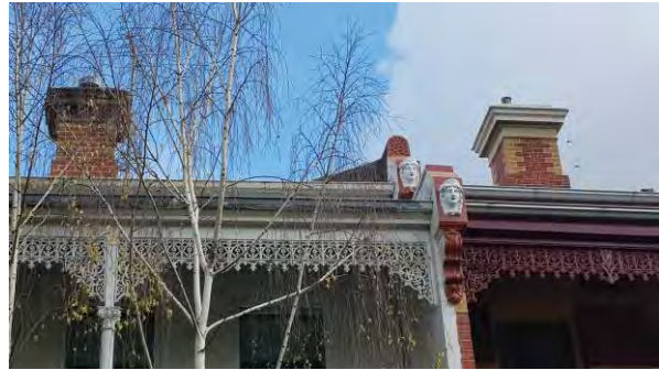
Figure 470. Detail showing decorative fascias, corbels and Italianate chimneys between Nos 547 and 549. (Source: GML Heritage, 2022)
