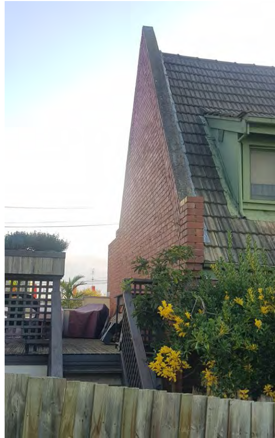
Figure 53. Detail showing the southern elevation and the adjoining deck of the neighbouring property. (Source: GML Heritage, 2022)
