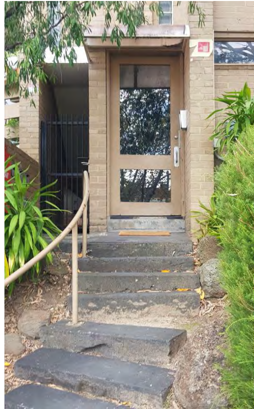
Figure 97. Detail of a primary doorway and stone steps with a contemporary railing leading to the rear carpark. (Source: GML Heritage, 2022)
