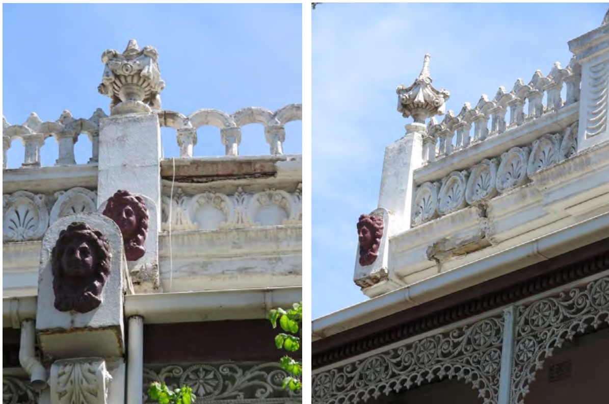
Figure Different building programs used slightly different parapet decoration (at left); parapet at no 199 (at right); note spalling render throughout
