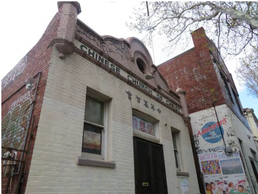
Figure 2 Detail of the principal facade, note the overpainted brickwork and distinctive parapet and pediment Source: Lovell Chen, 2022
