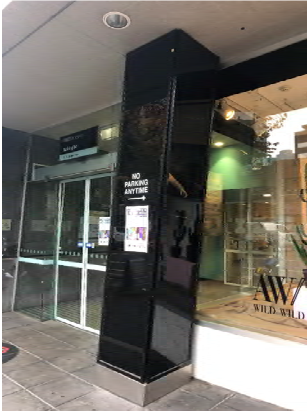
Figure 13 Detail of tilted column, recessed ground floor to northern bay Source: Lovell Chen
