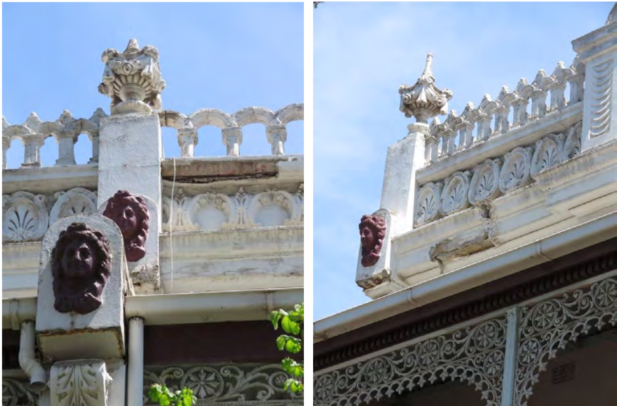
Figure Different building programs used slightly different parapet decoration (at left); parapet at no 199 (at right); note spalling render throughout
