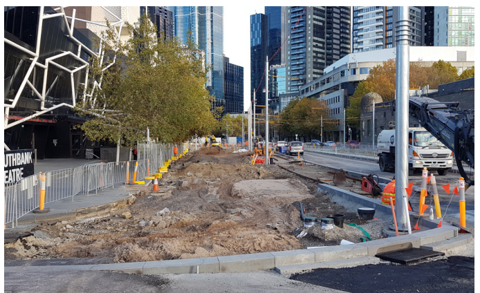
Works have commenced on Stage 2 - the first of the landscape spaces to the front of the Melbourne Recital Centre and Southbank Theatre.
