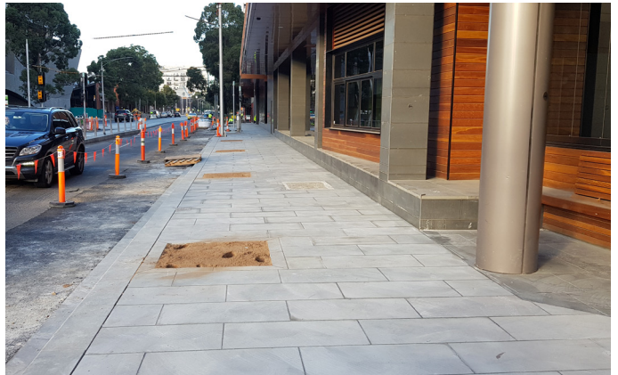
Bluestone footpaths along Southbank Boulevard and Sturt Street are being progressively completed and opened.
