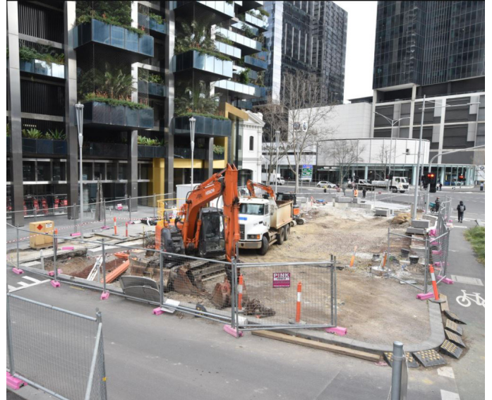
Work continues on the neighbourhood park between Fawkner Street and City Road
