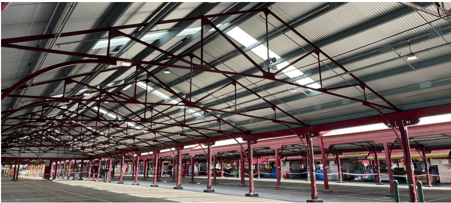
Photo: The newly restored C Shed ready to welcome A and B traders
