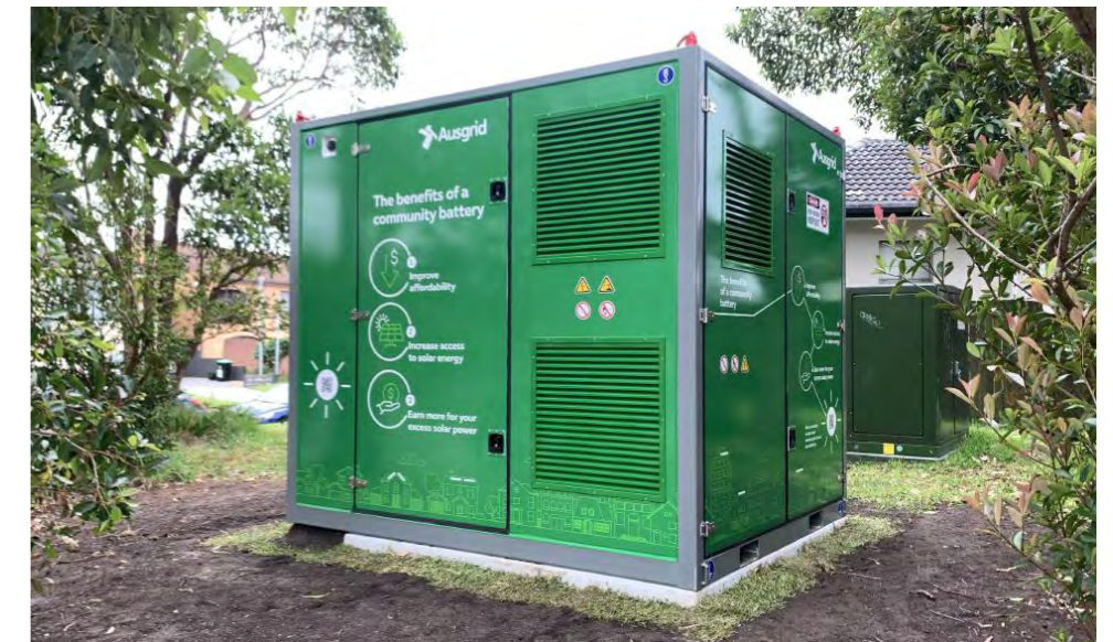
Beacon Hill community battery. Photography by Nadine Morton
