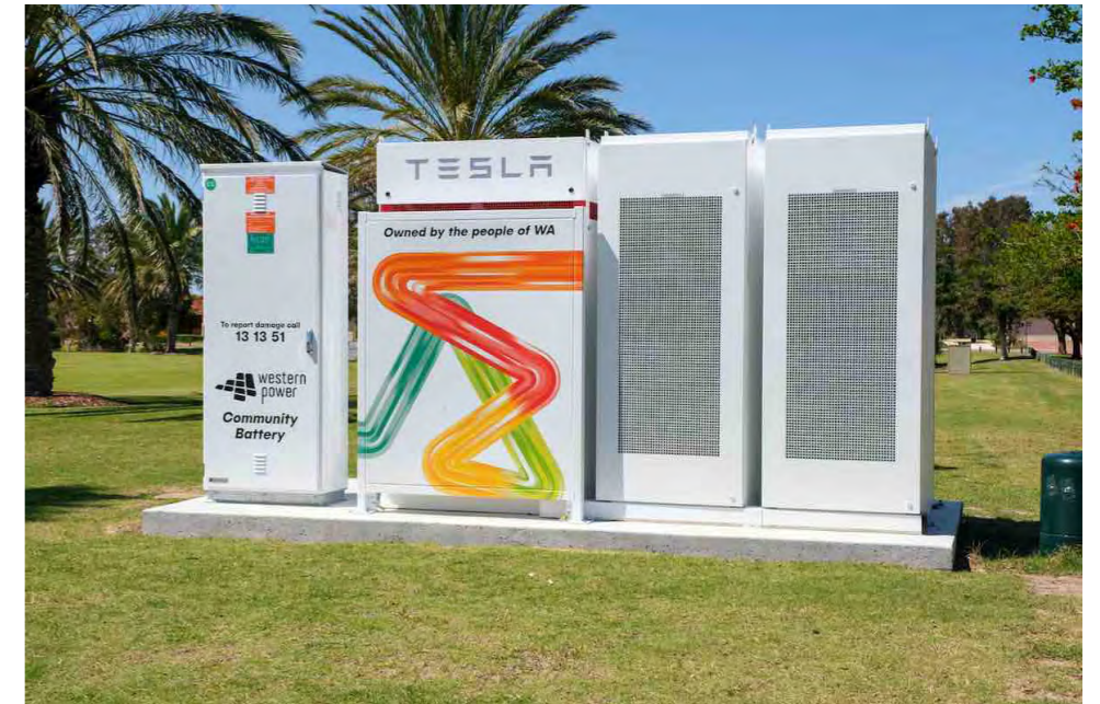
Community battery installed at Port Kennedy as part of a WA trial. Photo sourced from onestepoffthegrid.com.au
