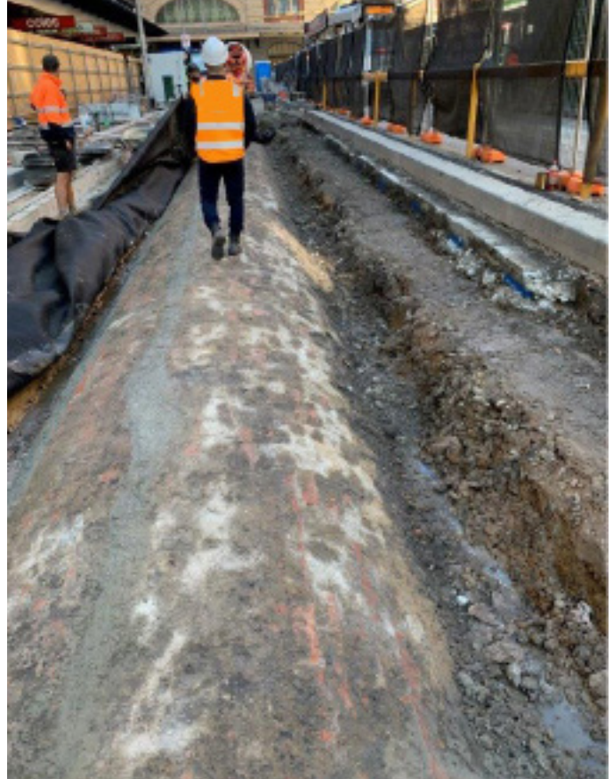
Exposed 120-year-old brick drain
