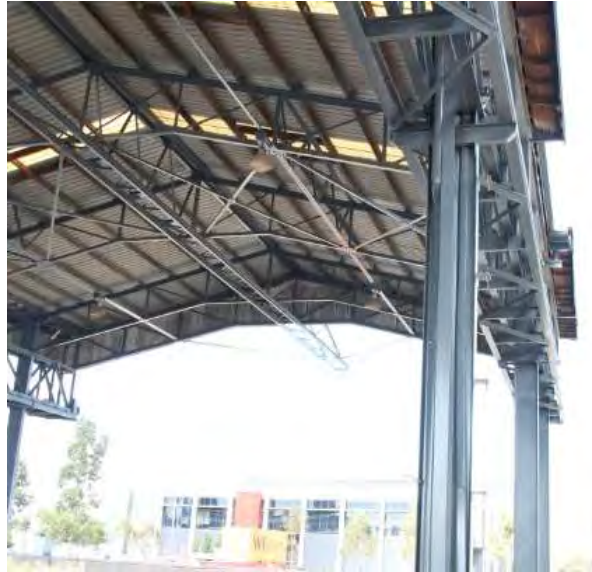
Figure 8: The tray, supported on the cambered part of the roof truss, still extends to the south over the truck loading bay and provides evidence of the electrical supply. Original light fittings are still evident. (P Mills, 03/04/2018)
