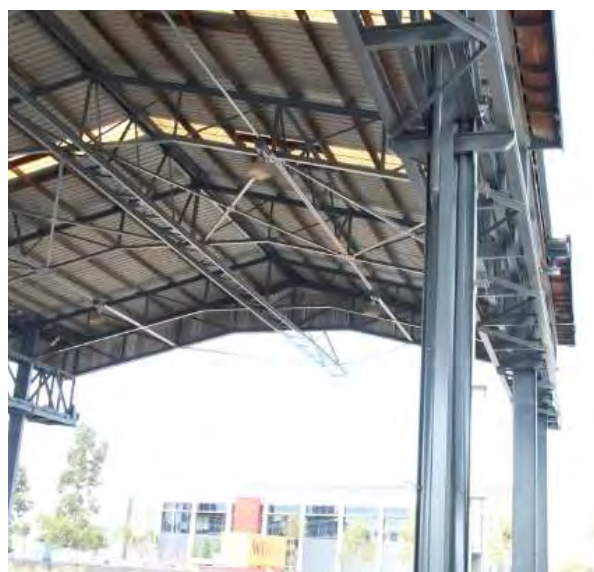
Figure 8: The tray, supported on the cambered part of the roof truss, still extends to the south over the truck loading bay and provides evidence of the electrical supply. Original light fittings are still evident. (P Mills, 03/04/2018)
