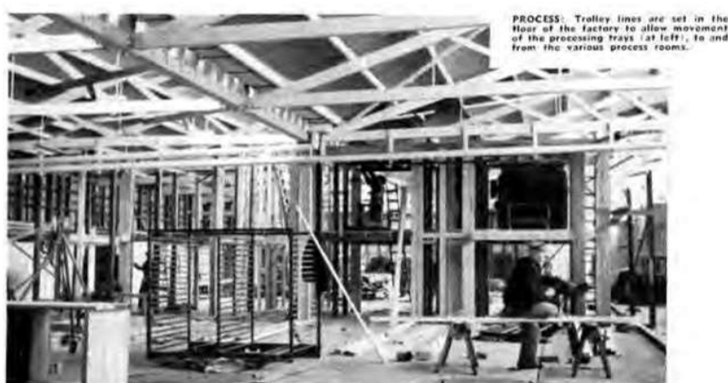
Figure 4: The Fishermans Bend dehydration factory interior under construction 1943 (Allied Works Council, 1943, p.74).
