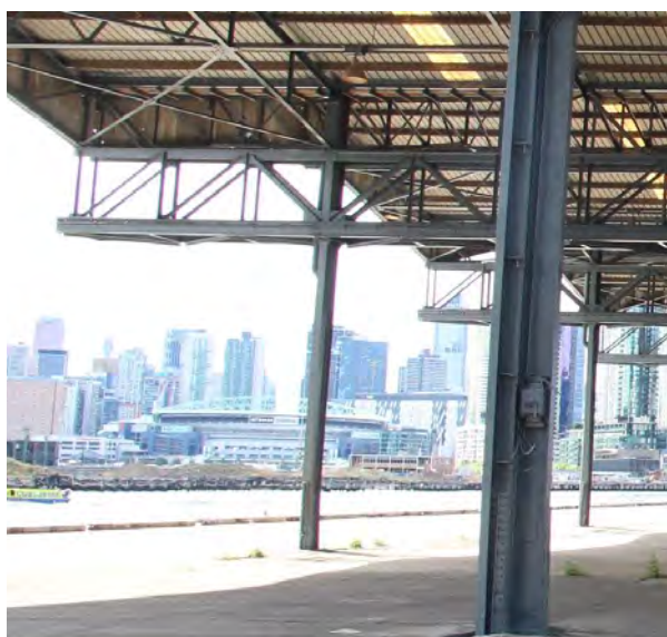
Figure 7: The flat, parallel chord trusses originally extended past the building towards the river and were supported on columns but have now been cut off. They supported the seven bridge cranes which have been removed. The reinforced extension of the columns can be seen near the base. (P Mills, 03/04/2018)
