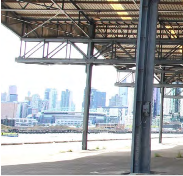
Figure 7: The flat, parallel chord trusses originally extended past the building towards the river and were supported on columns but have now been cut off. They supported the seven bridge cranes which have been removed. The reinforced extension of the columns can be seen near the base. (P Mills, 03/04/2018)
