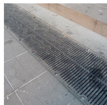
Examples of pits, covers & grates
