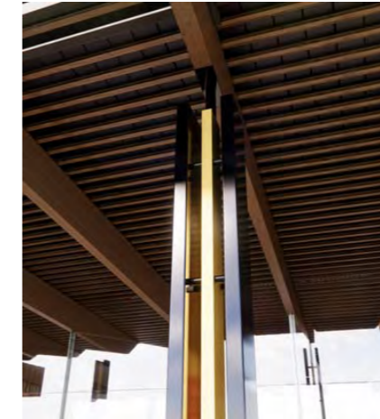
COL2 DUAL CHARCOAL POWDERCOAT STEEL RHS W/ PAINTED YELLOW RHS INSERT. BRACED BY WELDED STEEL RODS.
