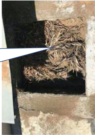
Grevillea leaves clogging roof gutter downpipe
