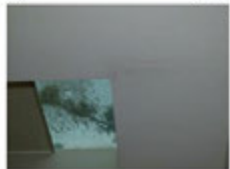
ceiling leak location.jpg 170K
