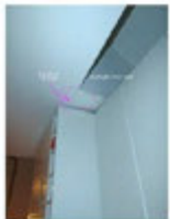
location of kitchen ceiling leak.jpg 1648K
