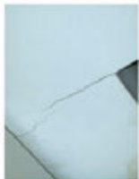
ceiling leak closeup 1.jpg 2775K
