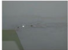
water drop from leak.jpg 244K
