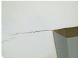
ceiling leak closeup 2.jpg 2686K
