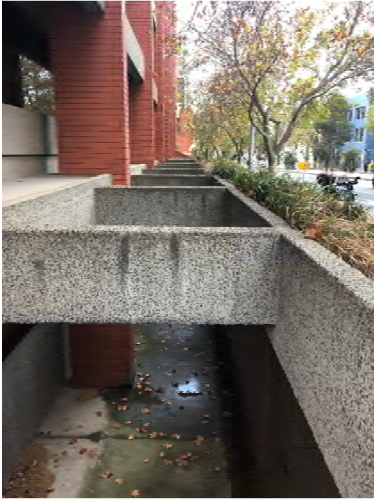
Figure 11 Building 56, north side, detail of lightwell to basement level below Source: Lovell Chen
