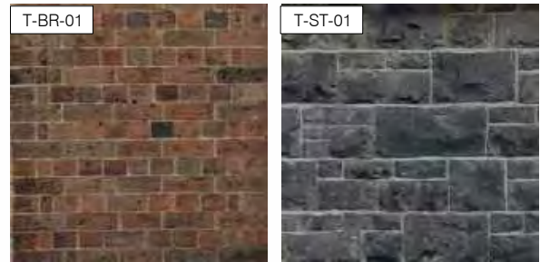
T-BR-01 Restored brickwork to 364 Albert Street (Eastern Elevation) T-ST-01 Restored bluestone to 364 Albert Street (Eastern Elevation)
