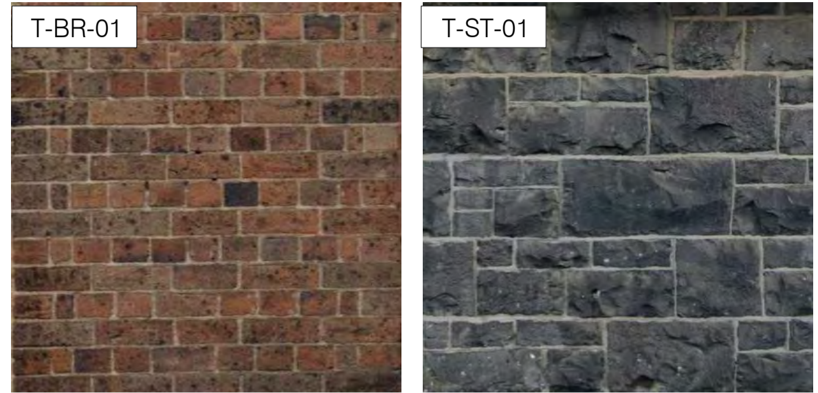
T-BR-01 Restored brickwork to 364 Albert Street (Eastern Elevation) T-ST-01 Restored bluestone to 364 Albert Street (Eastern Elevation)
