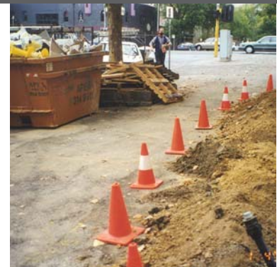
Site materials should not spill onto paths and solid hoardings should be used.
