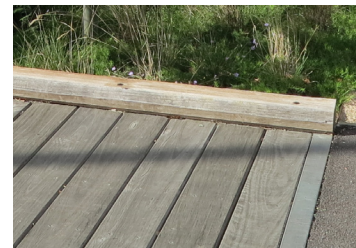
Timber deck bridge with timber edges - used at Royal Park over swales
