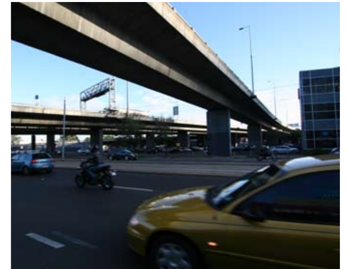
2.17.A Westgate Freeway & Kings Way condition
