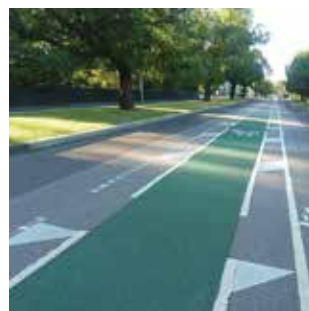
Double chevron bike lane markings
