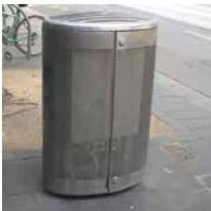
DESIGN STANDARDS: Examples of an electrical cabinet
