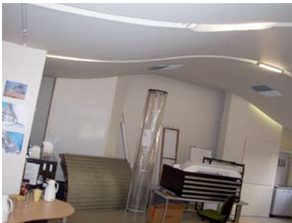
Figure 1. Mock up of the ceiling testing how differing elements will fit together
