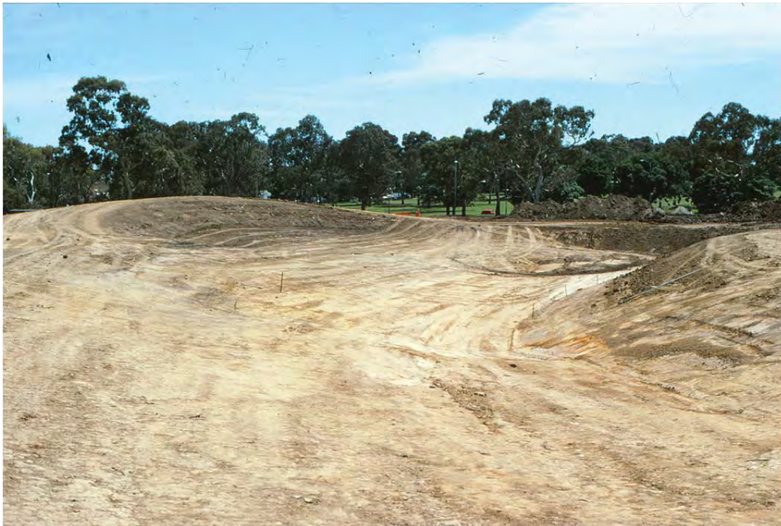
Royal Park, Stage II, Earthworks for the Hilbert Mound and the large pool (now known as the Billabong) located at the corner of Flemington Road and Elliott Avenue. November 1989. Bruce Cartwright
