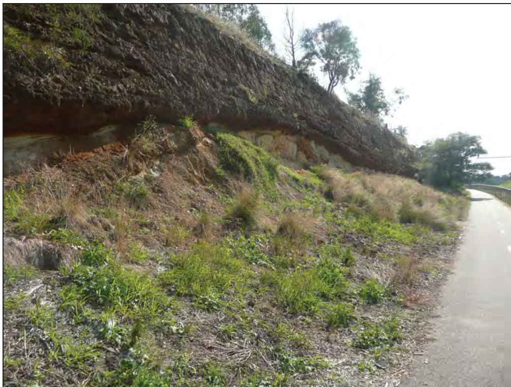
Plate 6. Section of railway embankment, 2010. Exotic vegetation with some planting adjacent to cycle path.
