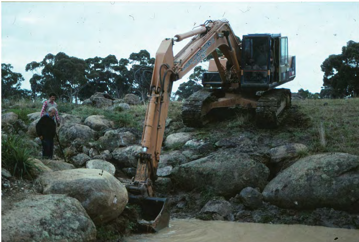
Royal Park: Stage II. Reinstating rockwork for the pool, April 1991. Bruce Cartwright
