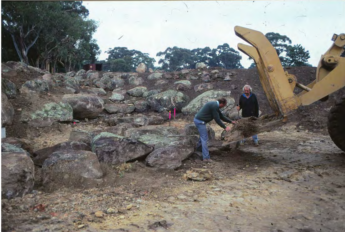
Royal Park: Stage II. Placement of the boulders for the pool, March 1990. Bruce Cartwright
