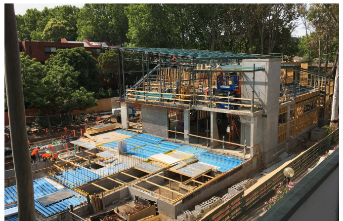
December 2019 – Sub-floor insulation and preparation for ground floor slab (front of site)
