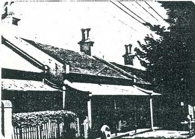
Low pitched slate roofs without front parapets were a common early Victorian feature prior to the use of elaborate decoration in the later Victorian period. The chimneys provide a uniform punctuation and are capped by tall terra cotta chimney pots. The use of a concave profile verandah roof was very common in this period.
